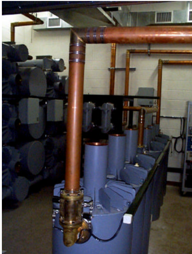
Figure 9 WMGC-FM Auxiliary Antenna Combiner
