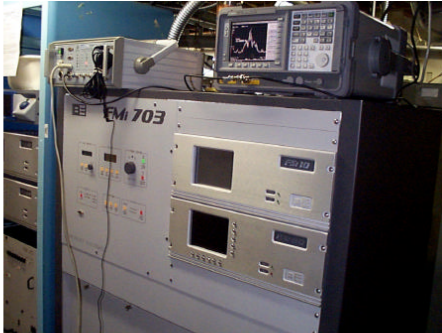
Figure 12 KDFC-FM Broadcast Electronics FMi 703 IBOC Transmitter
