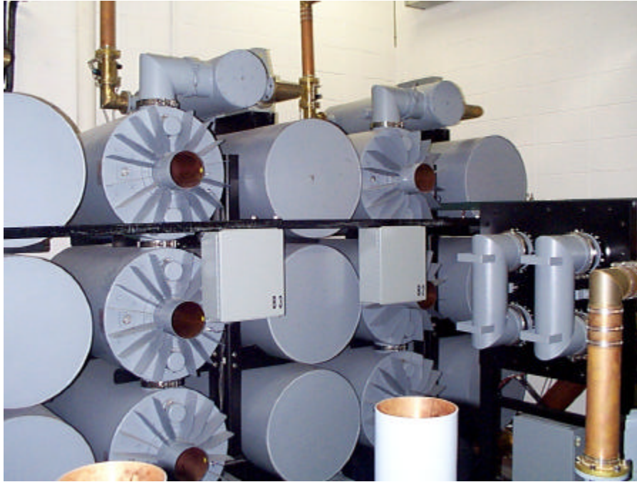
Figure 8 WMGC-FM Main Antenna Combiner
